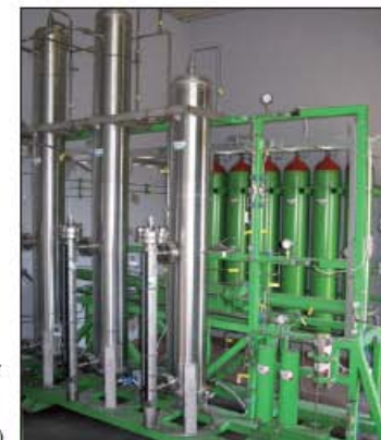
Figure 1. The patented Metener biogas upgrading technology (Jussi Lantela, Metener Ltd.)
